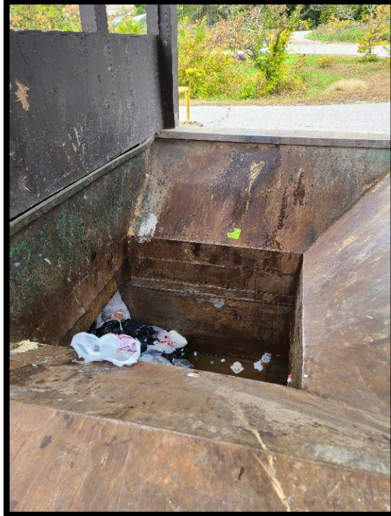
Photo 21: MSW Compactor Hopper
