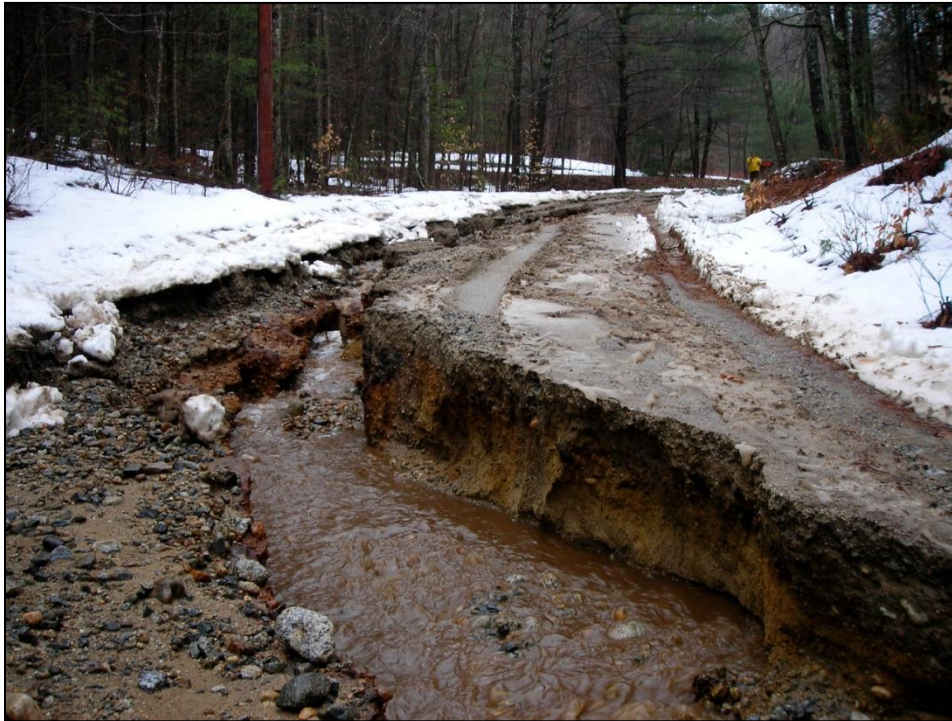
Howe Lane Washout
