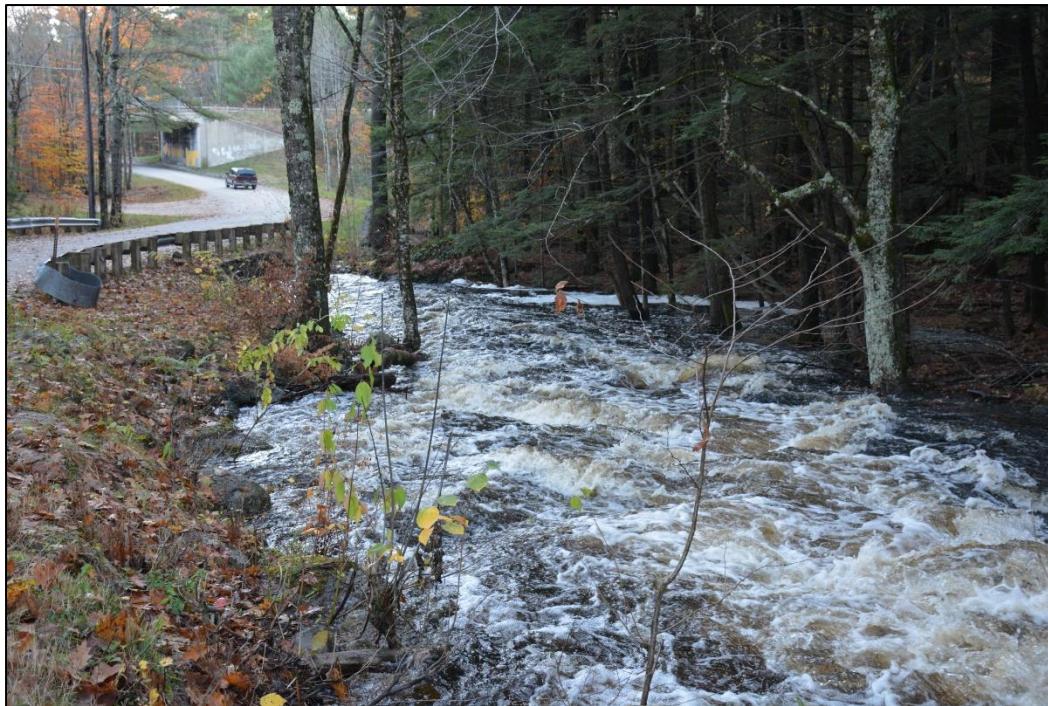
Flooded Stevens Brook along North Road (in Sutton), October 2017
