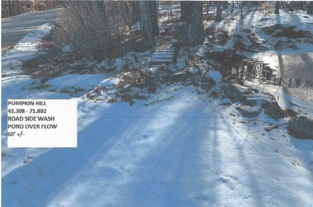
Roadside washout on Pumpkin Hill, from a combination of ground runoff and pond water overflow
