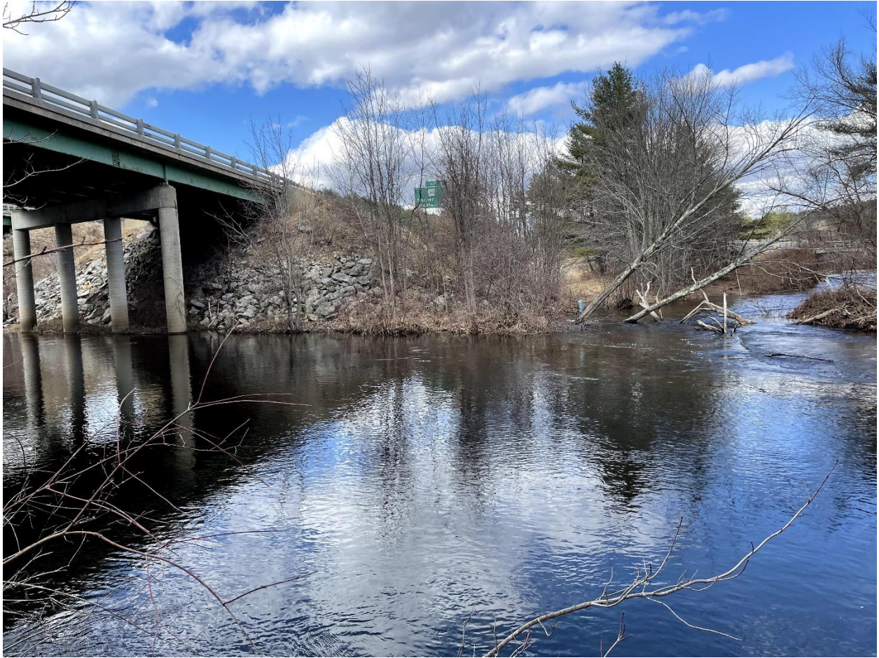
The warner River overflows near Exit 9. Photo courtesy of Tim Blagden
