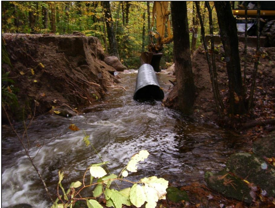
Culvert Washout on Ladd Lane
