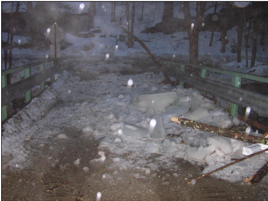
Laing Bridge Ice Jam and Debris Impacted Infrastructure (Warner River), January 2018
