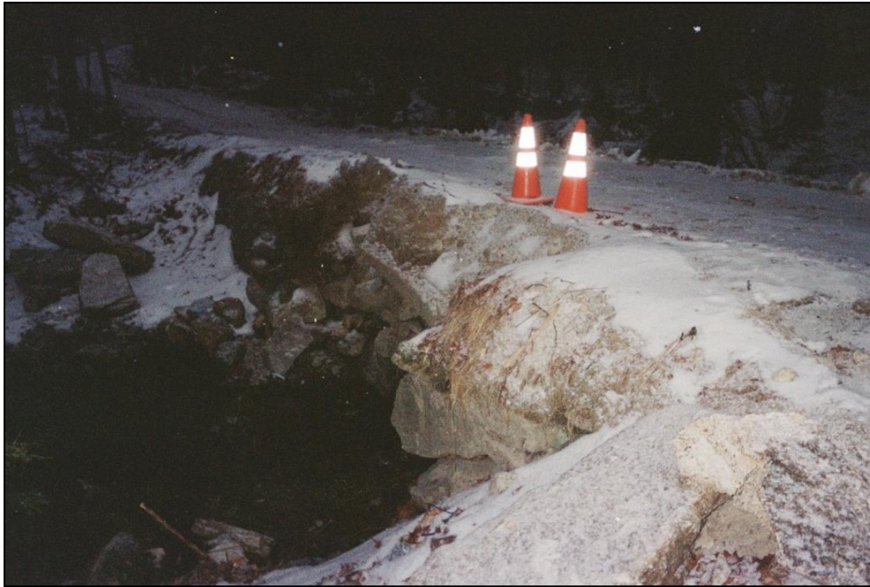
Unidentified Road and Culvert Icy Conditions, December 2008
