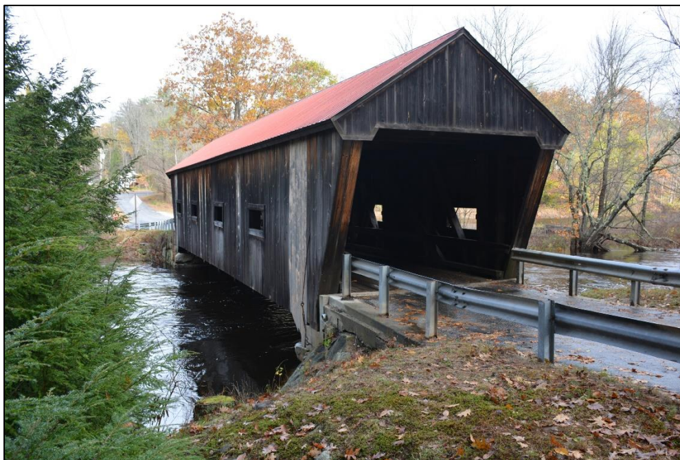
Flooded Warner River under Dalton Covered Bridge/West Joppa Road, October 2017
